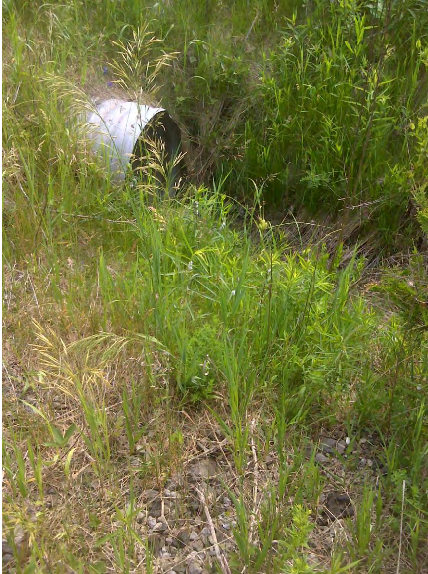
Figure 4-10: WA11 Drainage ditch along north side of Taylor-Kidd Road
